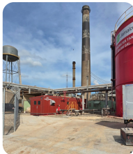
Firewater system pumphouse unit
