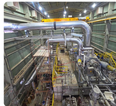
Interior view of Turbine Generator 4
