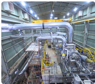
A peek inside the generator
