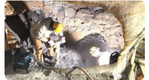
Employees of Contractor FC Reynolds descending the Cone of the furnace during the Calciner Overhaul.
