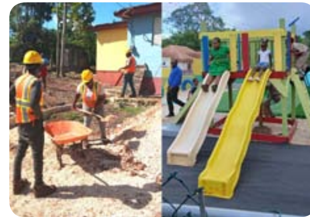
Photo at left shows workmen building the play area, while photo at right shows students playing on the newly renovated play area at the Victoria Town Primary School.
