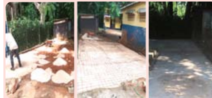
Photo at left and centre show the paving work partially complete, while photo at right shows the paved section of the schoolyard at the Porus Primary School.
